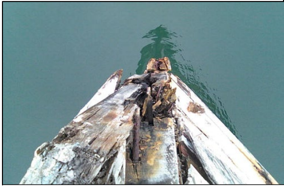
Extensive damage to the Petrel due to dry rot exposed after a minor collision with another boat. Photo submitted by John Kumparak.
